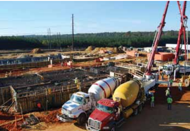
Construction begins on McIntosh Units 4 & 5, which will add an additional 360 megawatts of capacity when completed in 2010.
