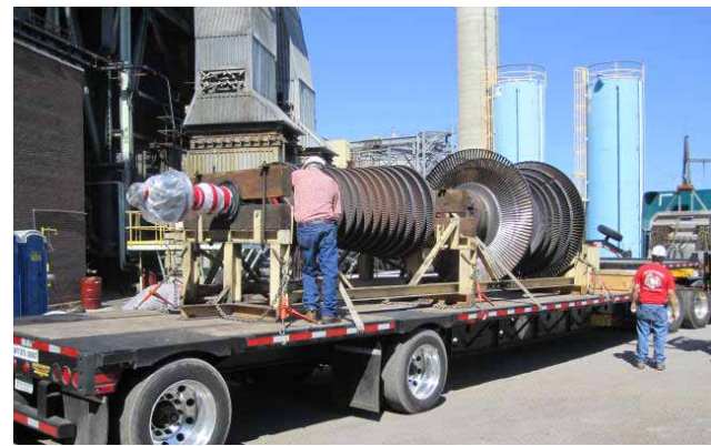
The rotor from Lowman's Unit 1 was removed as part of the Unit's major planned outage.
